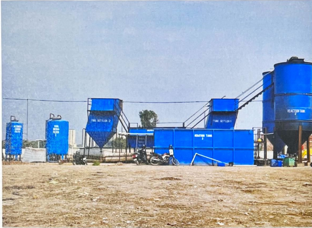
100 KLD LTP WITH COMPOST PLANT
